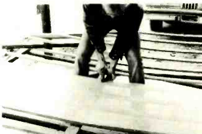
FIG. 15—KEEP TENSION ON THE SCREEN as you place the staples until you have tacked all around the edges. When working with the first strip of mesh you will have to stand between slats in the lattice.
